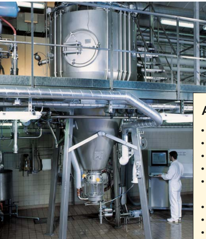
Integrated Filter Dryer operating at the Niro Test Station.
