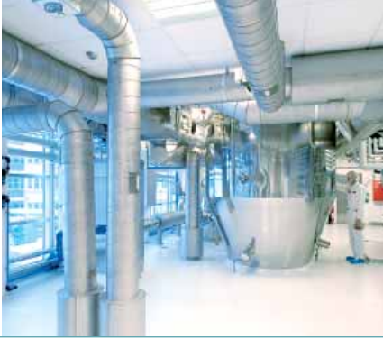
PSD-4 chamber and HVAC ducts
